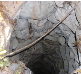
Open Well In Need of Closure: Potential for groundwater contamination and physical hazards.
